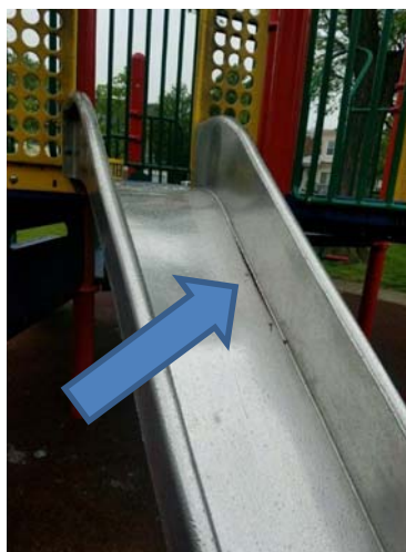
Arrow points to separated weld and gap between bedway and sidewall.
